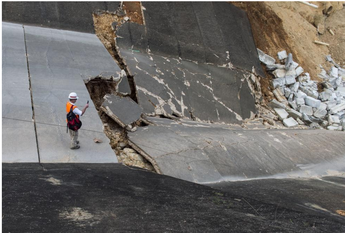
Hurricane Maria damaged the Guajataca Dam in September 2017 (Photo by Airman 1st Class Nicholas Dutton, 1st Combat Camera Squadron)
