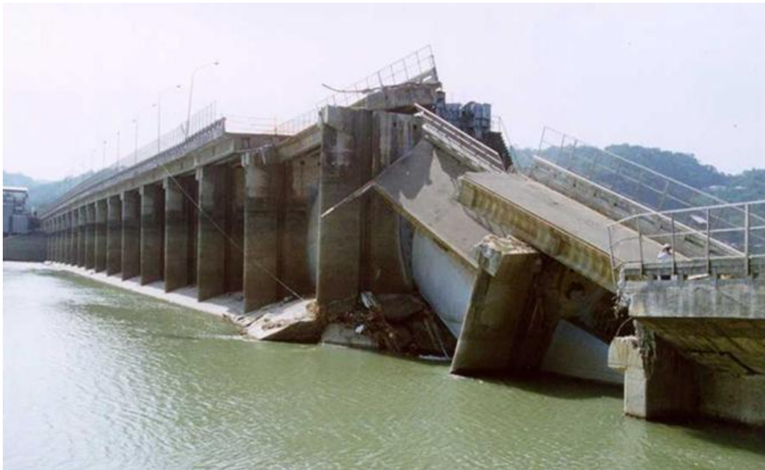
Shih-Kang Dam. Taiwan. Damaged by the magnitude 7.6 Chi-Chi earthquake on 21 September 1999 (Wieland, 2014)
